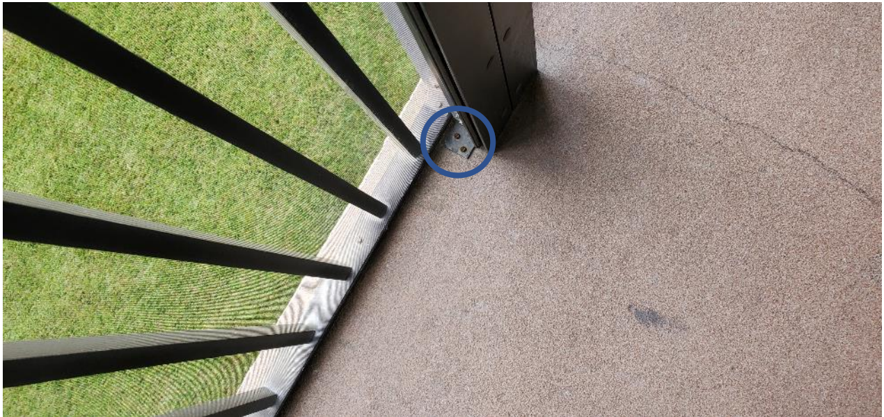
Corroded fasteners on shutter track
