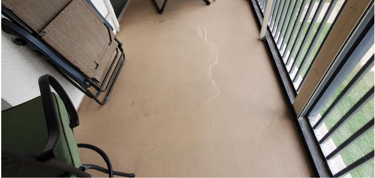
Concrete spall caused by reinforcing steel corrosion
