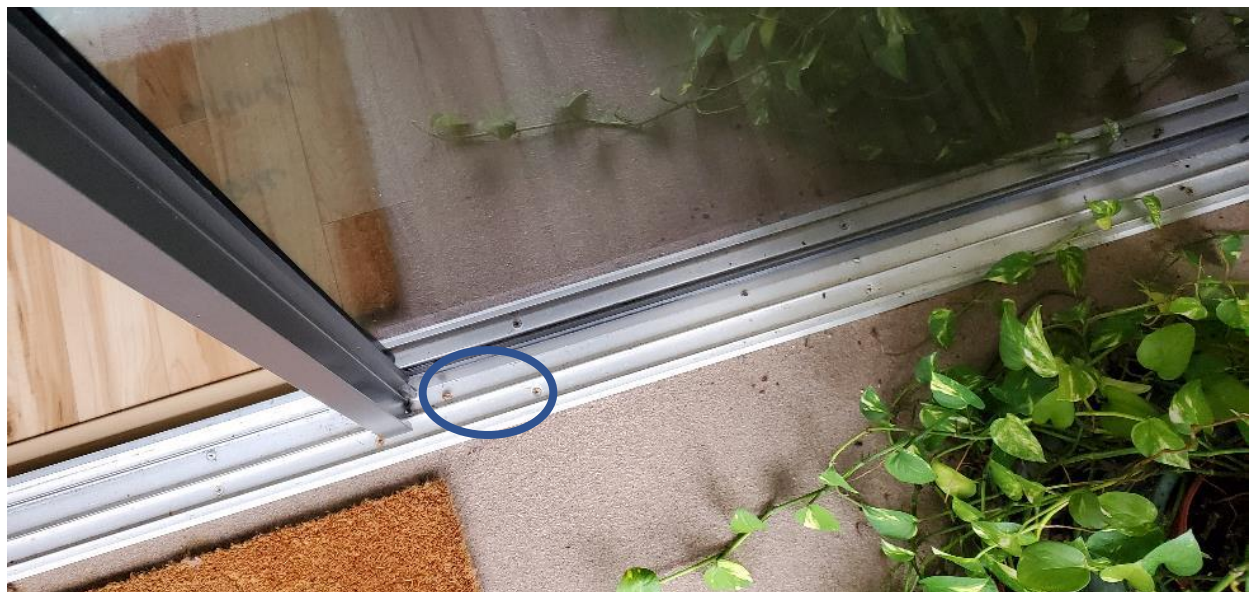
Corroded fasteners at sliding glass door
