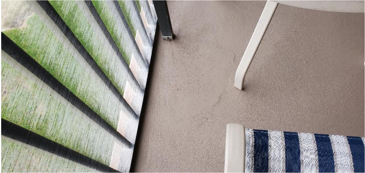
Spall along balcony slab edge, caused by reinforcing steel corrosion
