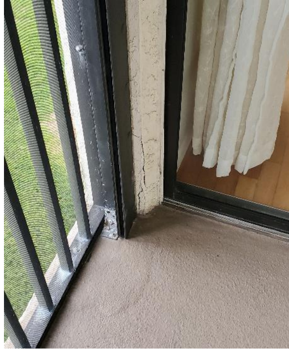
Column spall and edge spall caused by reinforcing steel corrosion
