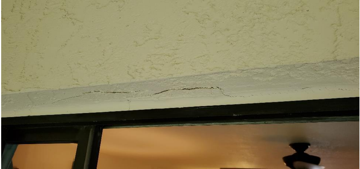
Cracks at sliding glass door header
