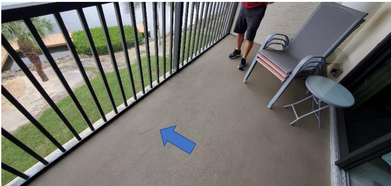
Spalls along balcony slab edge, caused by reinforcing steel corrosion
