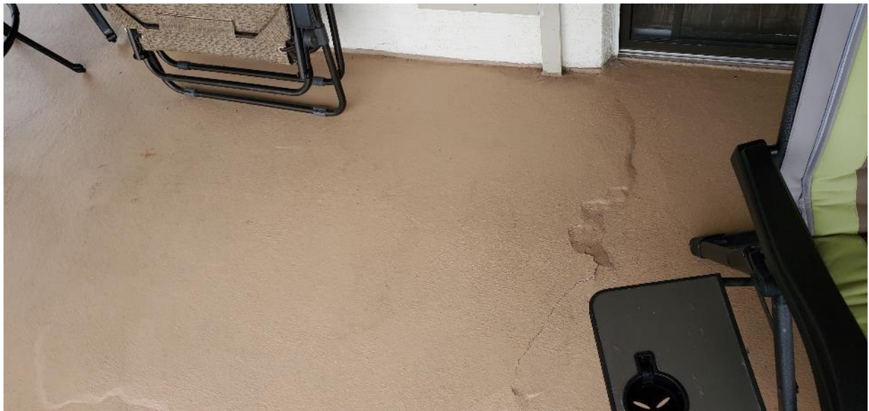
Advanced spall caused by reinforcing steel corrosion
