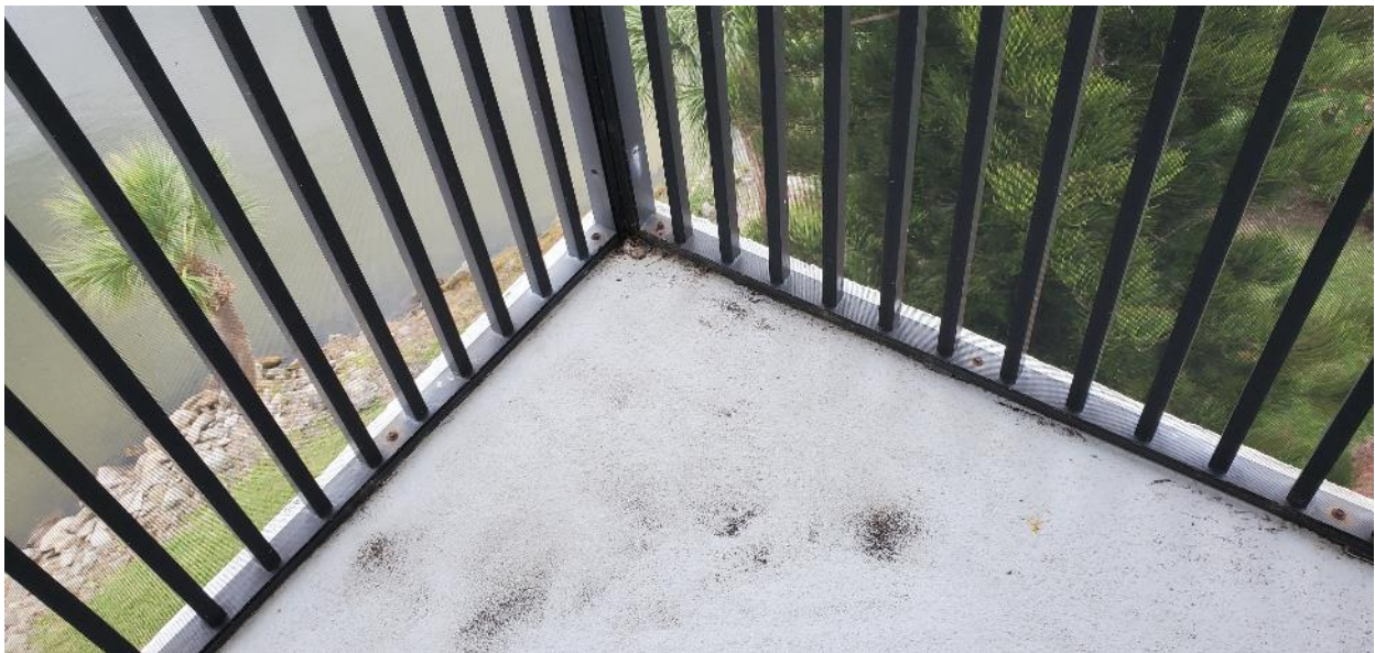
Corroded fasteners on screen enclosure
