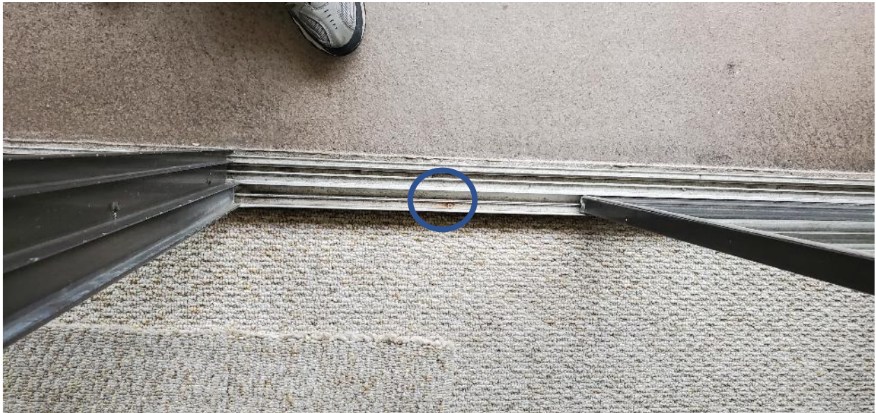
Corroded sliding glass door fasteners
