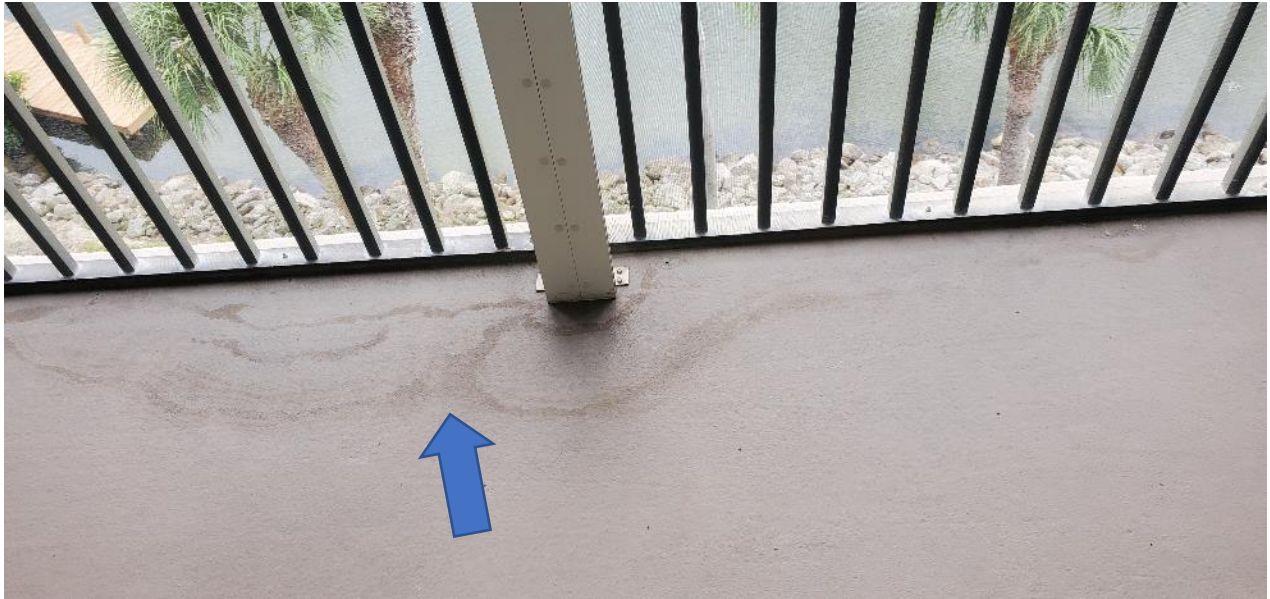
Ponding water evident from markings on balcony slab; screen enclosure/railings not shimmed
