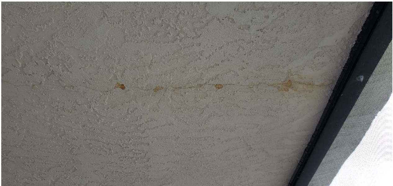
Cracks and rust spots on ceiling surface
