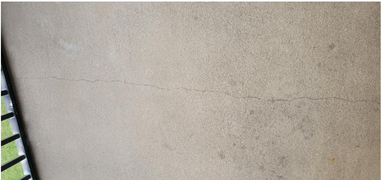
Cracks in balcony floor coating
