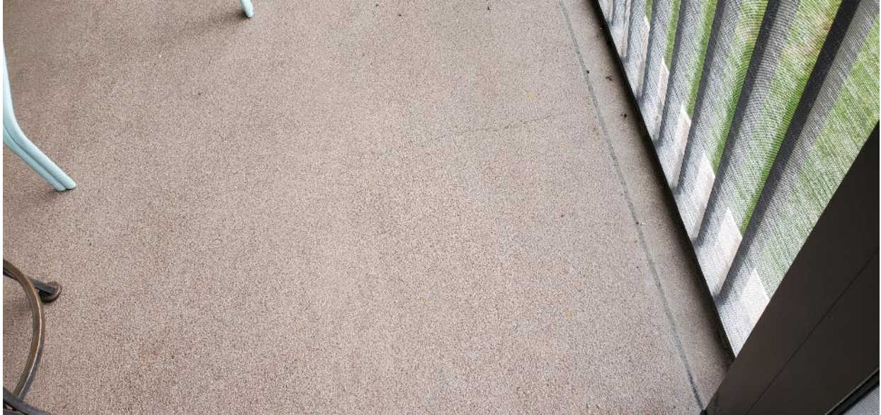
Cracks in balcony floor coating
