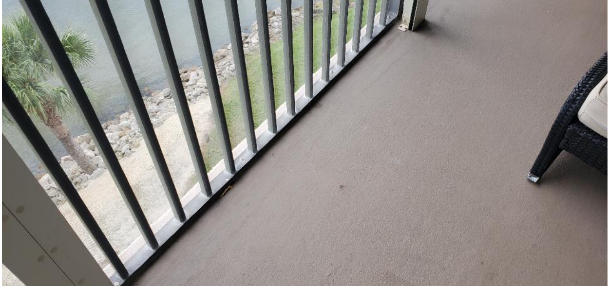
Screen enclosure/railing showing signs of oxidation
