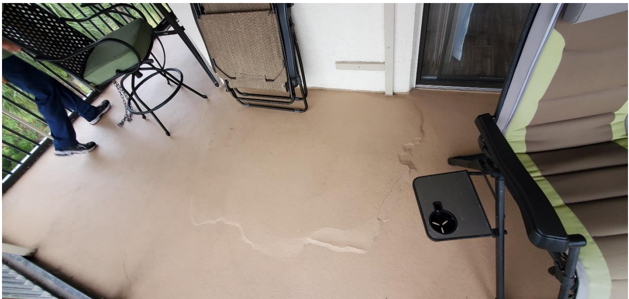
Concrete spall caused by reinforcing steel corrosion
