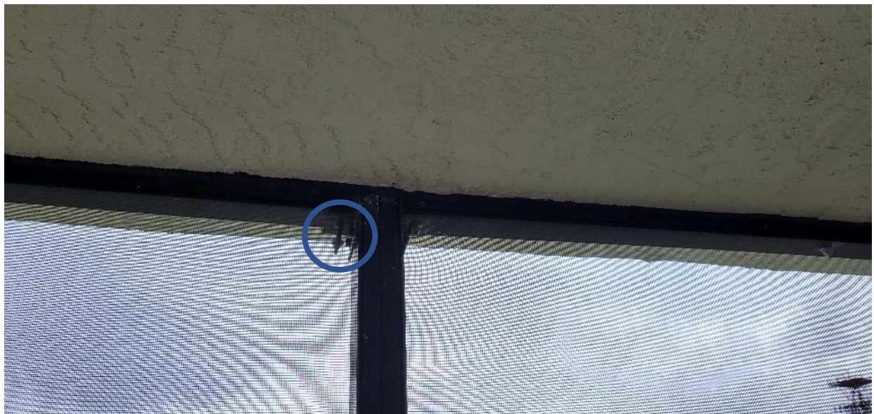
Screen enclosure fastener not embedded into concrete
