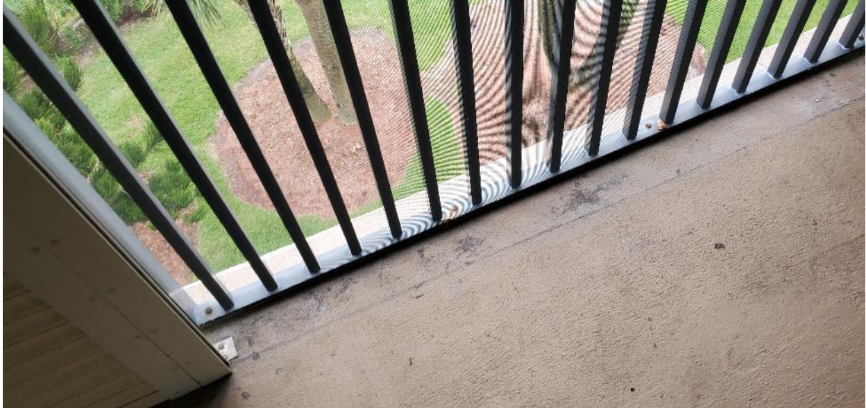
Corroded fasteners on screen enclosure
