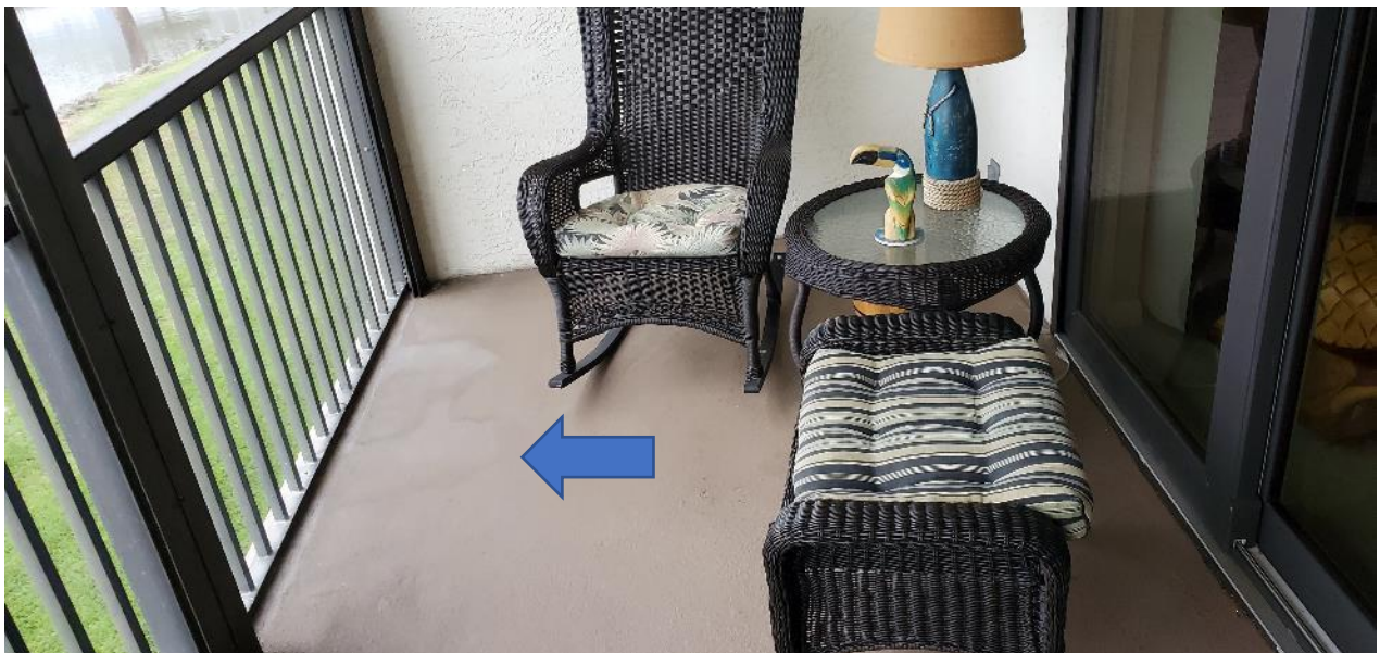
Ponding water evident from markings on balcony slab; screen enclosure/railings not shimmed
