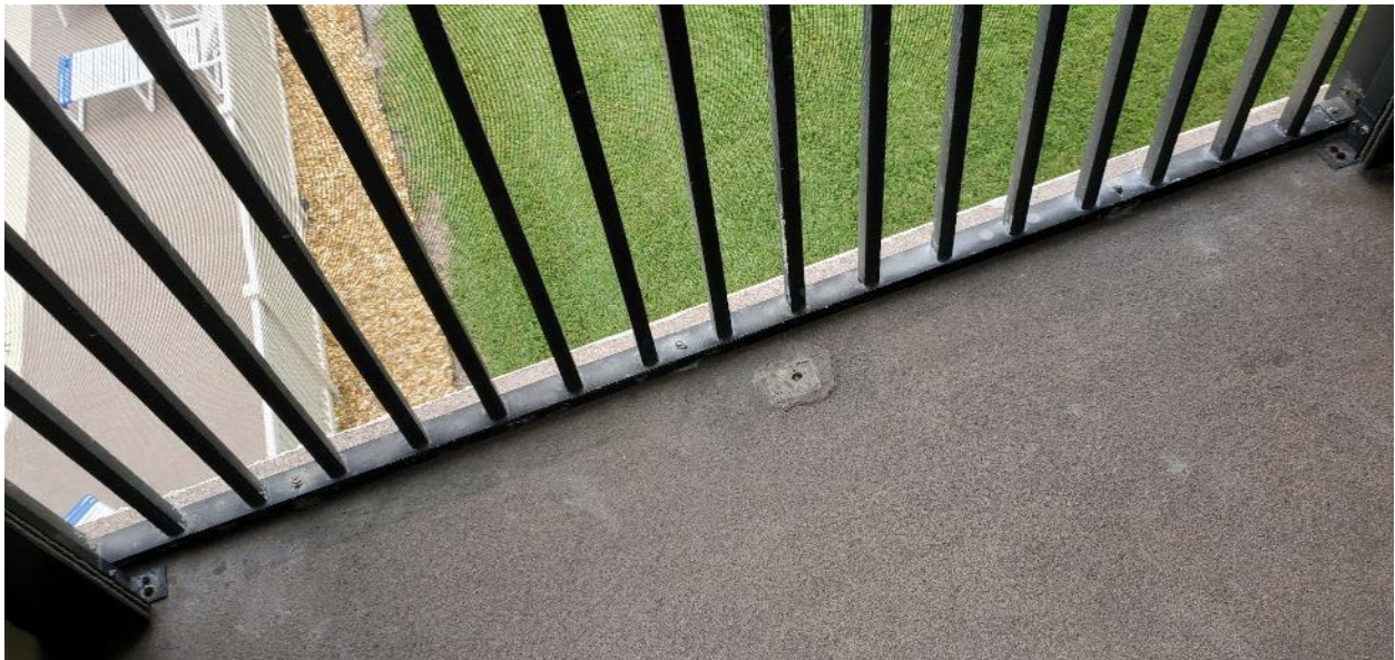
Enclosure/railing coating oxidizing and failing
