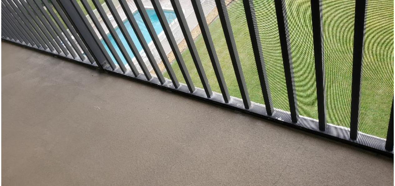
Enclosure/railing coating oxidizing and failing
