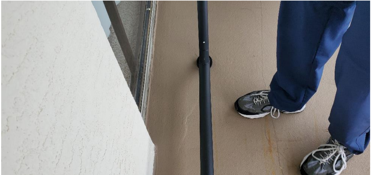
Concrete spall at sliding glass door caused by reinforcing steel corrosion
